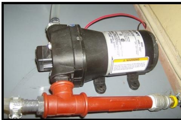
Figura 4.3 – Bomba y bypass
