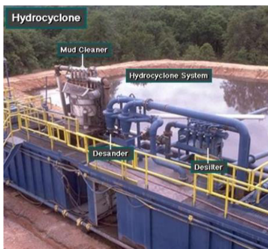
Figura # 61. Mud cleaner, desander y desilter.
