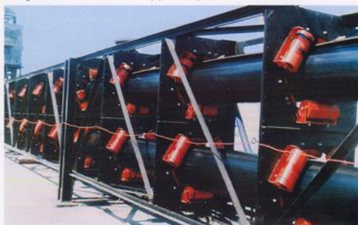
Fig. 3: Intermediate section of pipe conveyor
