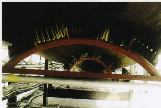
Fig. 2: Return Belt near tail end transition portion
