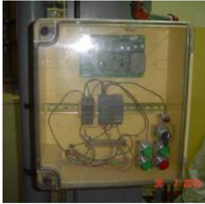
Panel de Control
