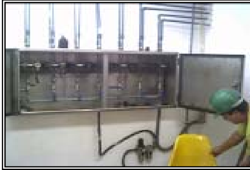
PANEL DE CONTROL NEUMATICO
