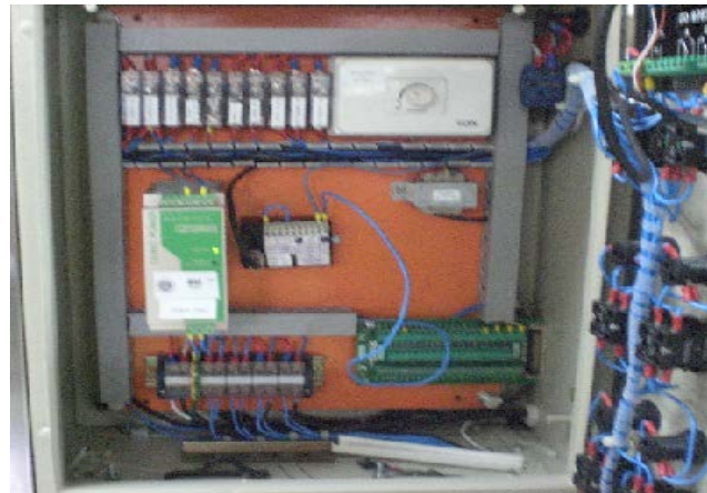
Figura 3.19 Vista Interior del panel de control
