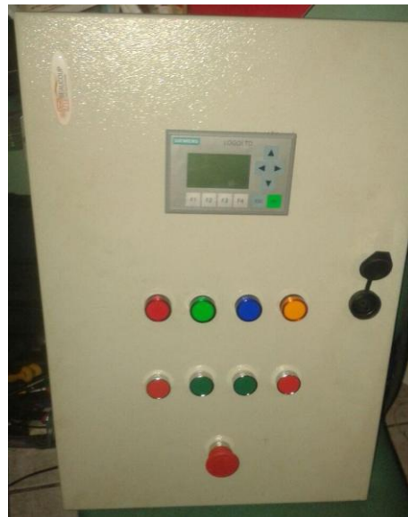
FIGURA 2.5: TABLERO DE CONTROL
