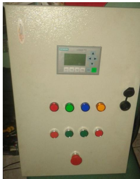
FIGURA 2.5: TABLERO DE CONTROL
