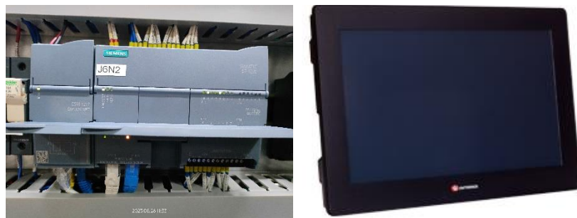
Figura 9.- PLC S7-1200 y HMI UNISTREAM.
