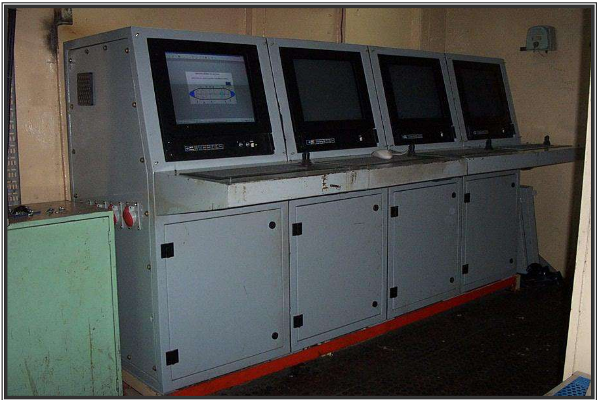
Figura No. 7.1 Consolas de Control
