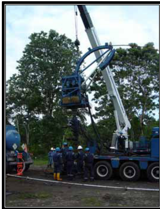
Figura 3.5 Unidad de Coilded Tubing
