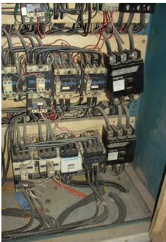
Fig. 12: Tablero de control [8]
