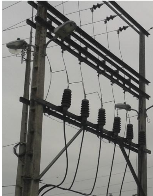
Figura 1.10 Patio de 13.8 KV
