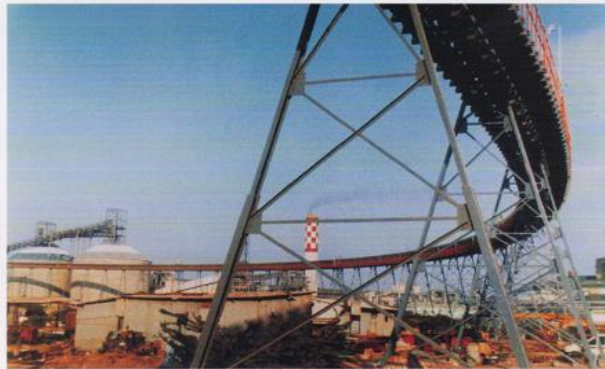
Fig.1: 3.2 km long pipe conveyor at Birla Copper
