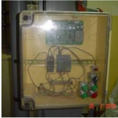
Panel de Control
