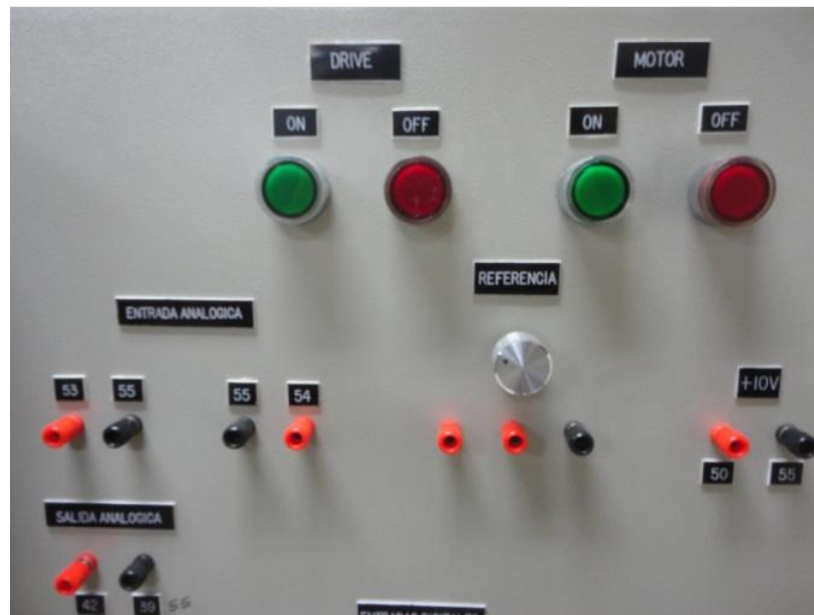
Figura 11.10: Vista superior del panel Danfoss.
