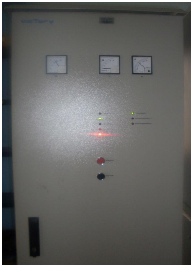
Figura 1.18 Panel de Alarma
