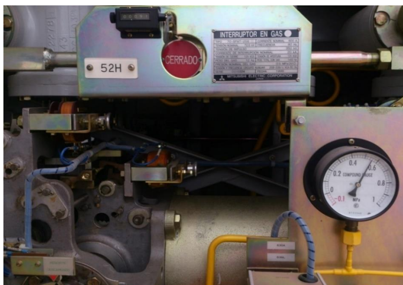
Figura 1.10 Interruptor Mitsubishi – lado 69 kV
