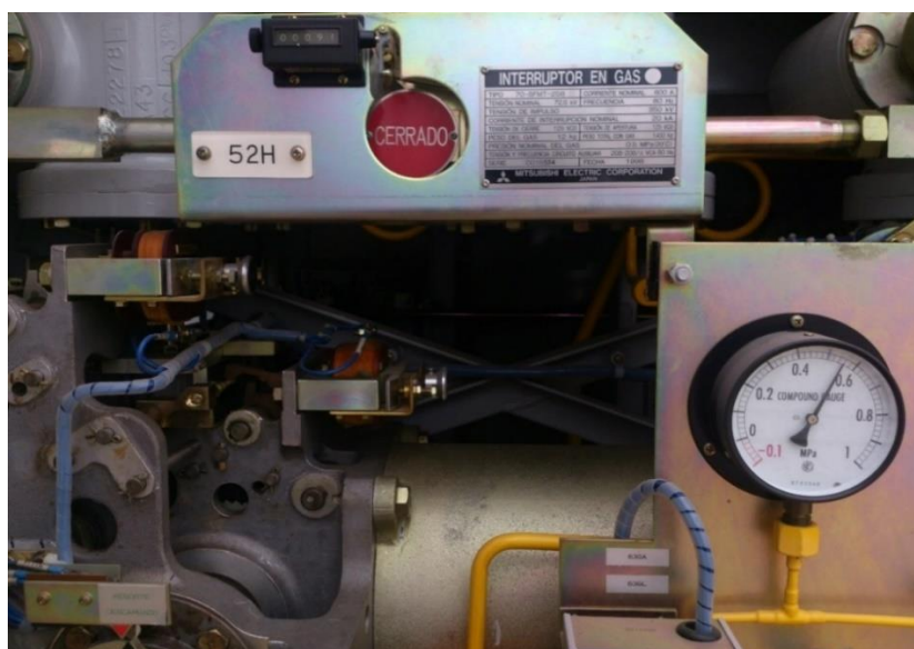
Figura 1.10 Interruptor Mitsubishi – lado 69 kV
