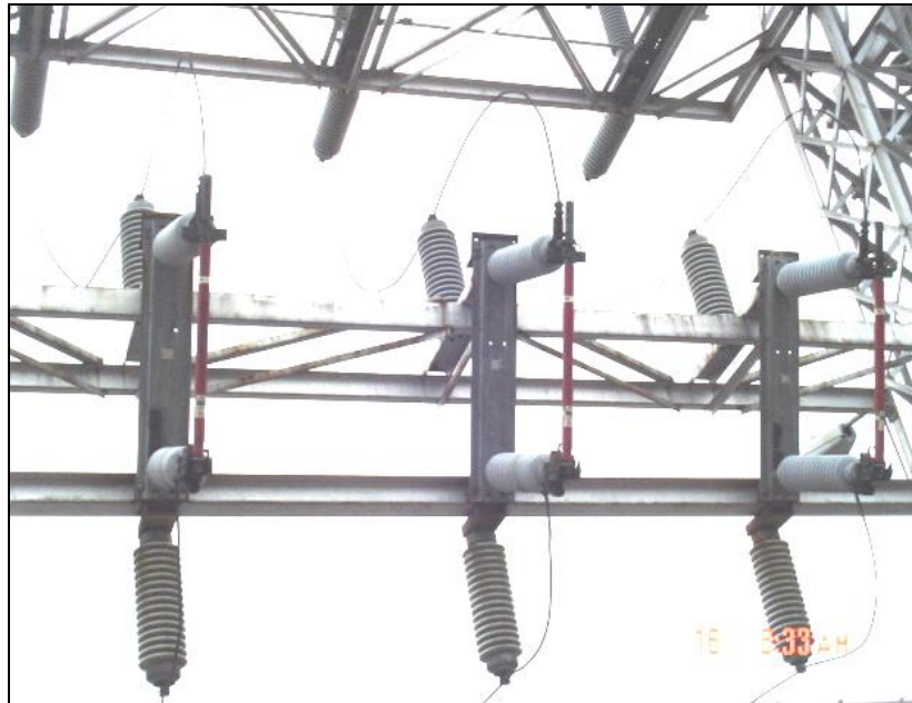
Fig. 4.4 Porta Fusibles – Fusibles
