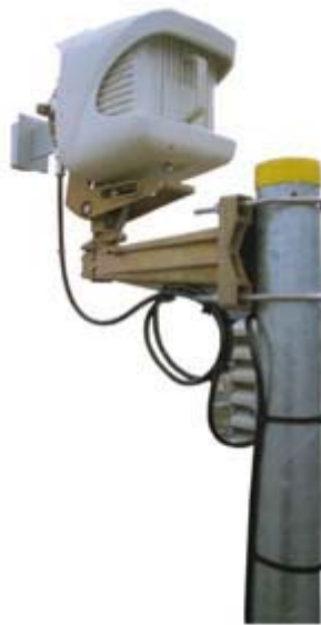
Figura 27. Radio Base Station
