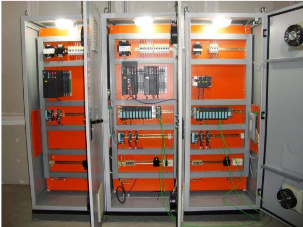
Figura 3.2: Tablero control central
