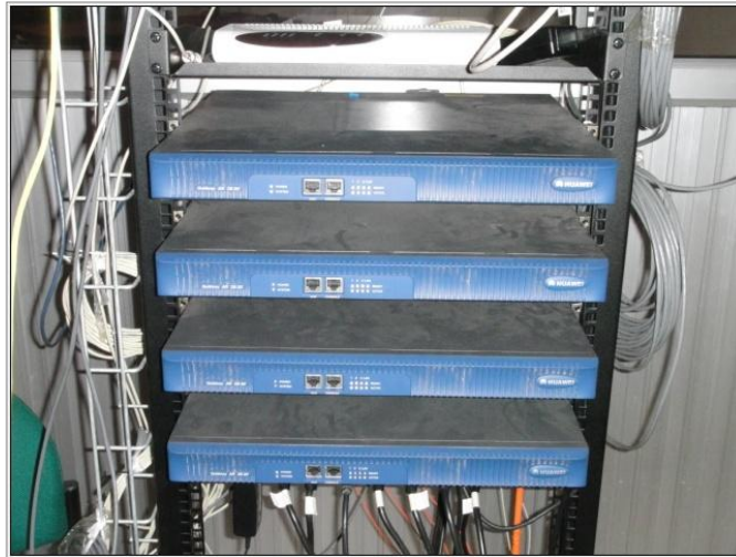
Figura 4.26.- Router HUAWEI QUIDWAY AR 28-30 [9]
