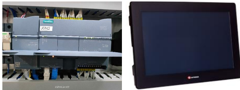
Figura 9.- PLC S7-1200 y HMI UNISTREAM.
