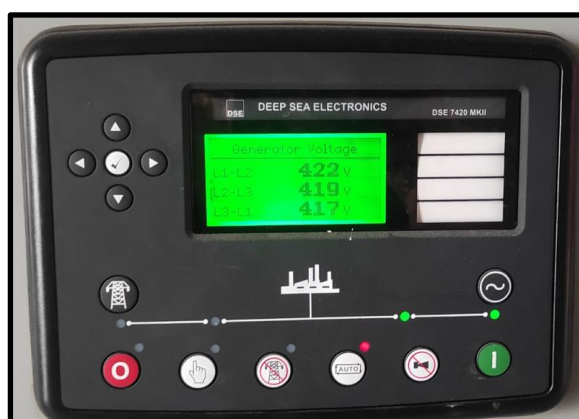
Figura 1.1 Modulo DeepSea Electronics 8610
