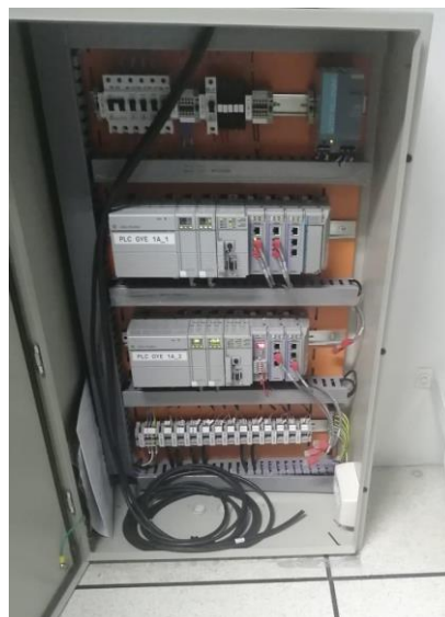
Figura 1.17 PLC compact Logix instalado
