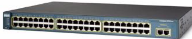
Figura.4.9.Switch Cisco catalyst 2950, 48 puertos
